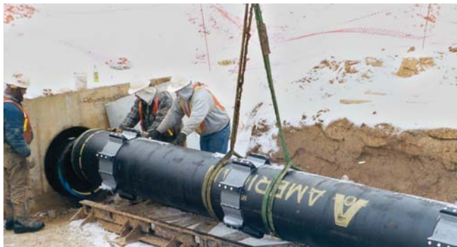
Model C12GN2 used on D.I Pipe, for 1,800 ft crossing under airport runway.
