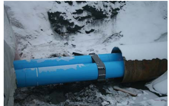
Model C12GN2 used on (2) 24" C-905 Chilled Water Lines going through a 60" casing.
